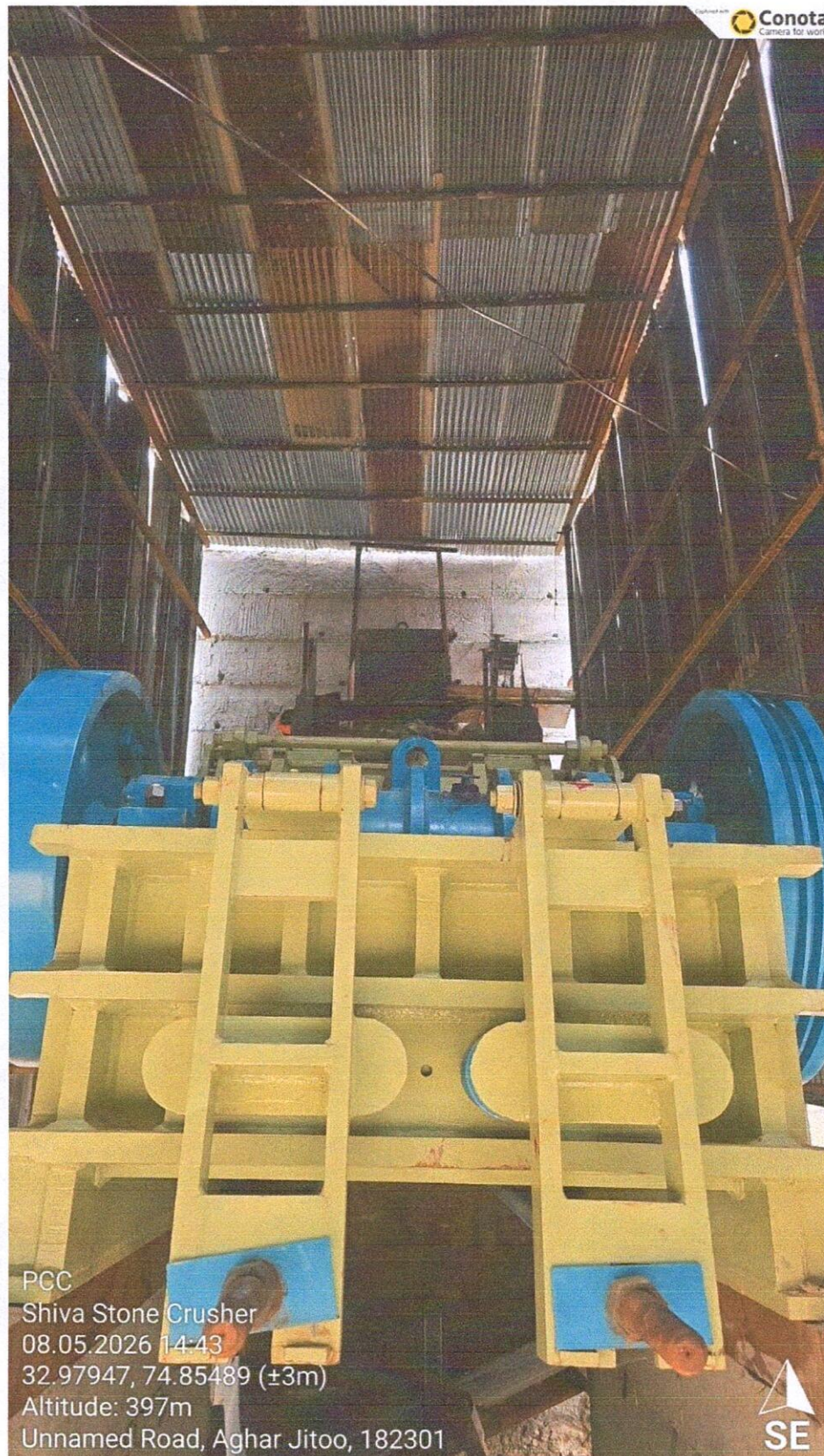
Pic-3: Sprinkling System installed at crushing point and is covered with GI Sheets.
